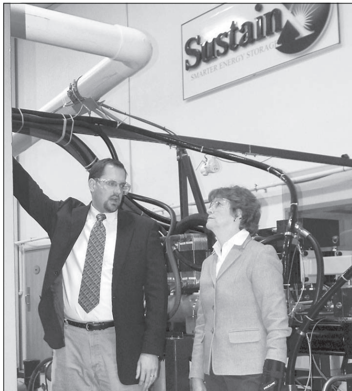
U.S. Sen. Jeanne Shaheen, D-NH, learns about SustainX's Isothermal Compressed Air Energy Storage pilot project from co-founder and director of systems engineering, Benjamin Bollinger, at the company's new facility in Seabrook on Wednesday.
